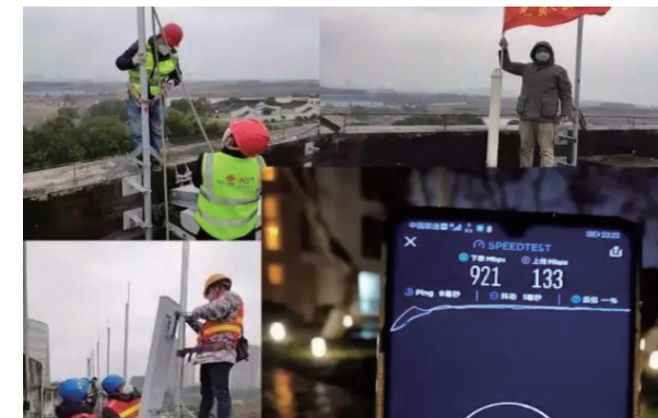
Figure 1: 5G network construction for Huoshenshan Hospital
